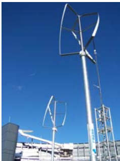
Turbines at the roof of the tower
